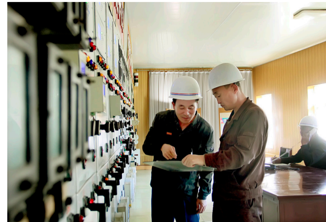
Technicians discuss how to improve the safety of the electric power system at the Nampho Municipal Power Distribution Station.
