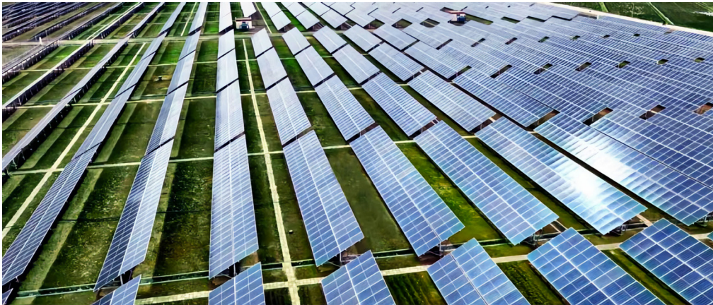
Newly built solar power plant in the City of Haeju, South Hwanghae Province.
